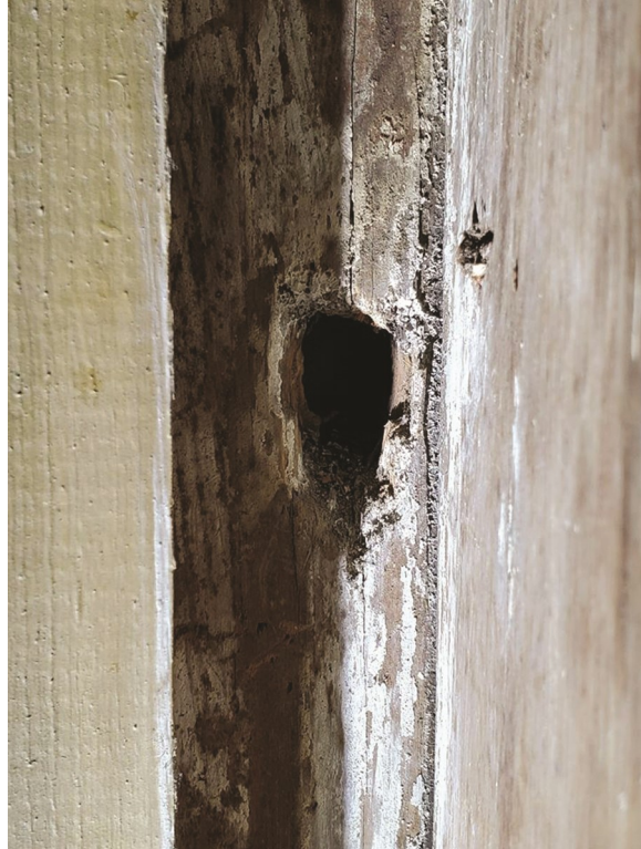
A new hole found near kitchen stairs. This hole was hidden when new molding was attached to the stairs leading into the cellar. It can be viewed only by looking along the wall on the reverse side with a flashlight.
