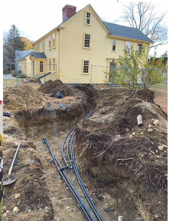
Tubes to carry liquid to geothermally heat and cool the Jason Russell House add an almost-futuristic dimension to the 1745 dwelling.
